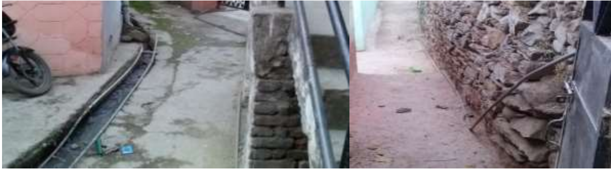
Figure 20: Water Supply Pipelines along Streets and Drains - Ramban Town (2014).
